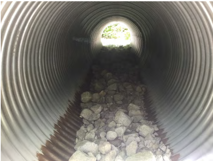
Aggrading in highchain culvert
